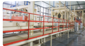
The production of Xingang Brand ultra-thin MDF has started, using the Yalian ultra-high speed Continuous flattening line machine, with an annual output of 200,000 m 3 .
